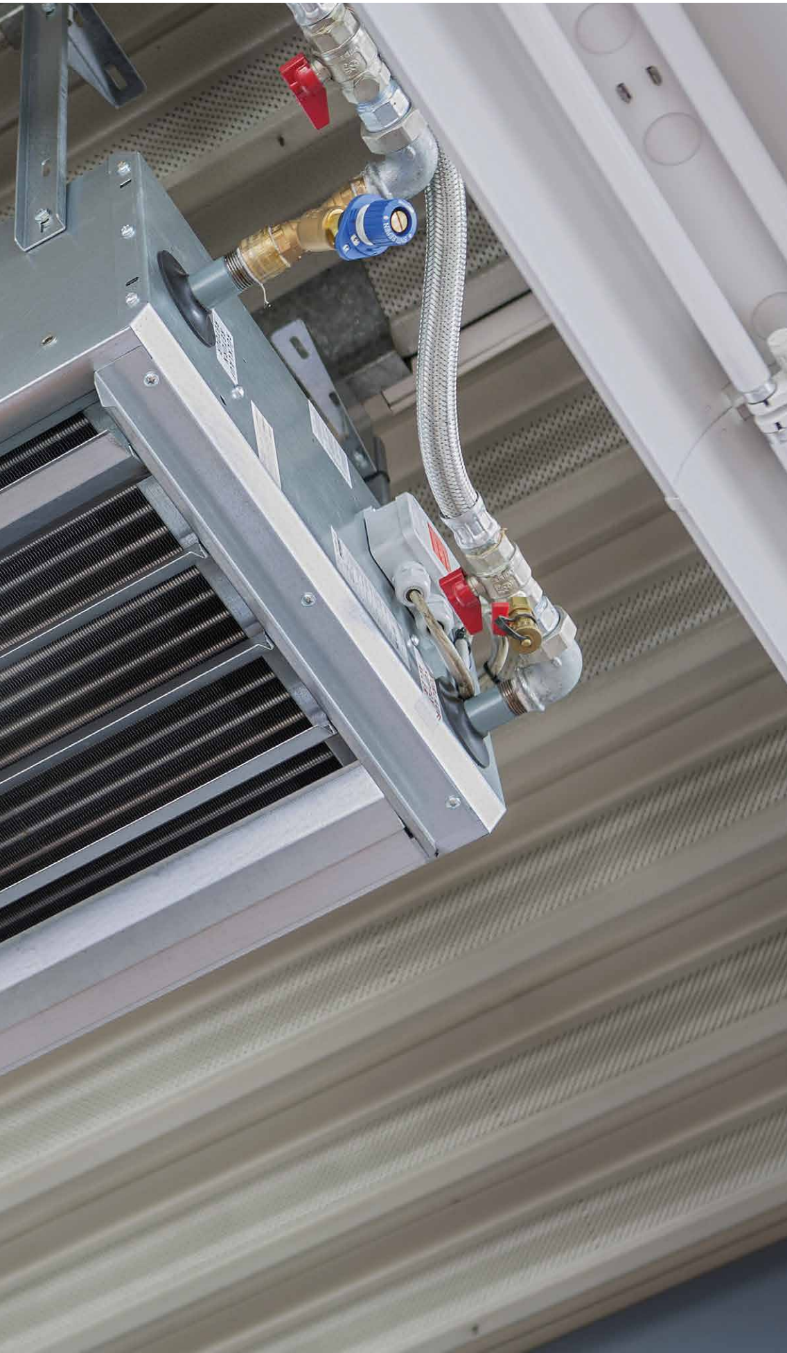
TIP unit heaters installed on the ceiling heat the showrooms belonging to the Seyfarth car dealership in Gotha.
